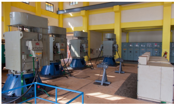
Raw water Pump House
